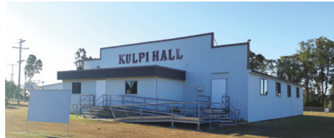
Kulpi Hall's new ramp providing better access for the all members of the community
